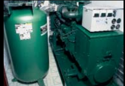
Optional Installed Generator, Air Compressor & A.C.
