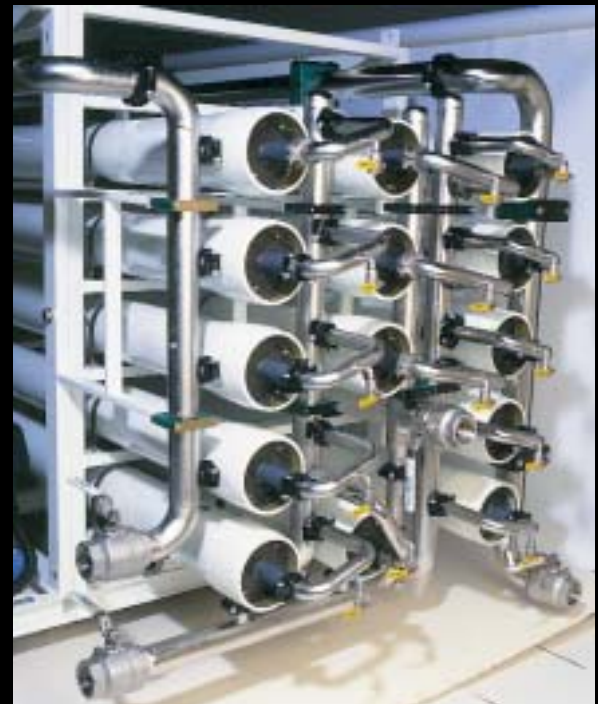
Stainless Steel HP Piping
